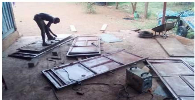
Welding of the doors for the secondary school block by the VTS students.
