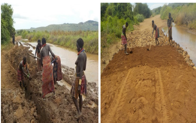
Scouring of the muddy road and filling of the potholes at the airstrip.
