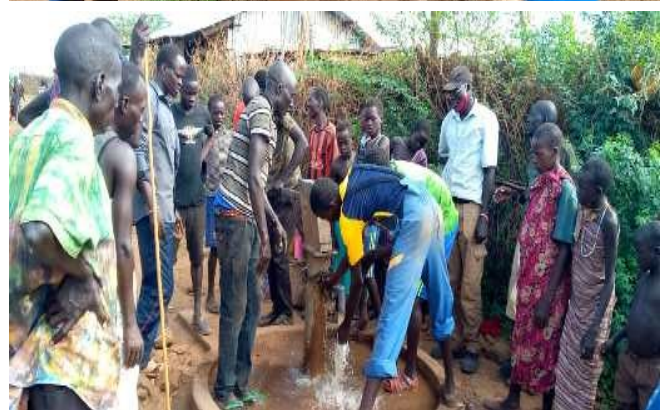
Rehabilitation of the community boreholes in the villages for clean drinking water and use of water during COVID-19
